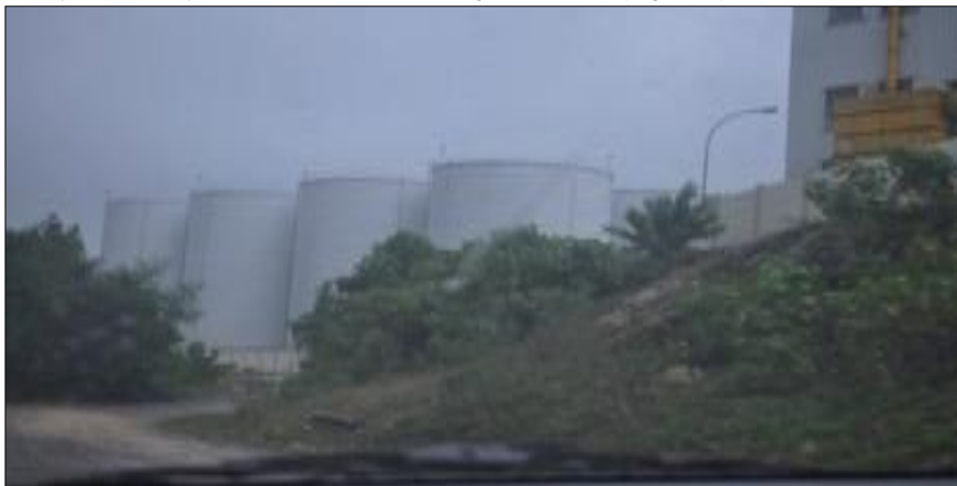
Figure 5. KPO and CPO storage tanks in the mills in North Mamuju
