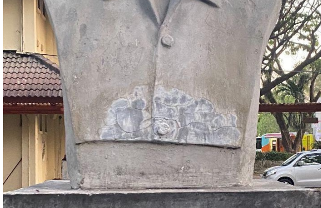
Figure 5. The appearance of cracks and efflorescence
