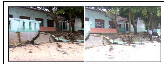
Figure 2. The condition of the coast behind SMAN 1 Lemong.
