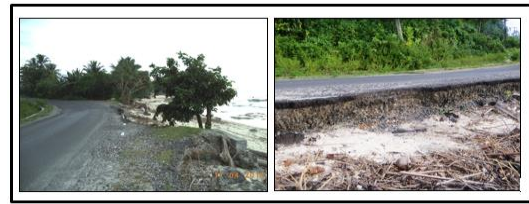
Figure 1. The condition of the west cross road in Lemong Sub-district has been affected by abrasion.
