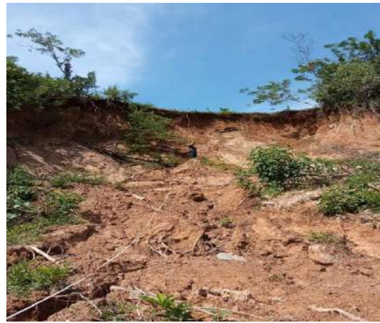
Figure 1. Documentation of the location of the North Bengkulu - Lebong crossing road that experienced a landslide on 26 March 2022.
