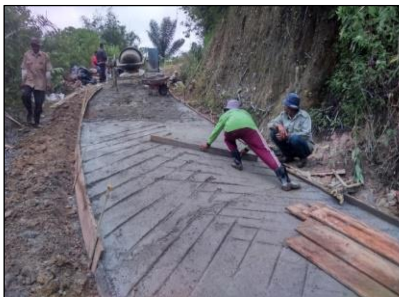
Figure 1. Road Repair in One of Jorong Nagari Tigo Balai (Sources: Authors Documentation, 2022)
