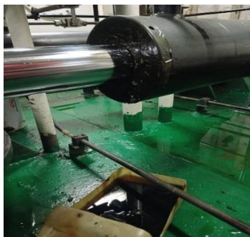
Fig.2. Leak in hydraulic cylinder
