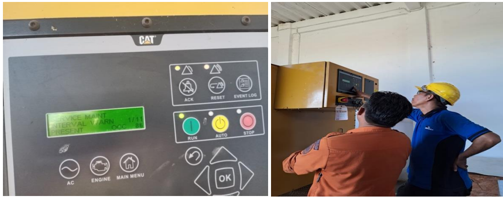
Figure 6. Indicator check by Trankindo technician
