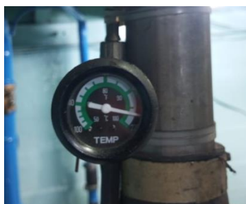
Figure 2. Freshwater Cooling System Temperature Measuring Instrument
